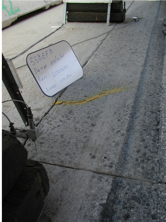
Figure 6.72. Close-up of first new crack after 2.002 million load repetitions.
