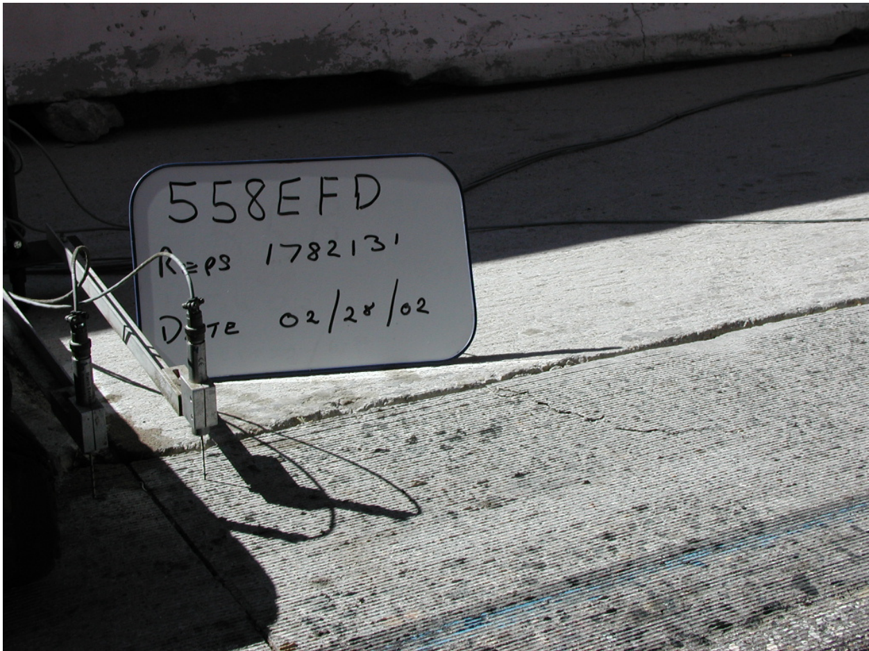
Figure 6.71. First new crack on Section 558FD from slab edge to back of outside dowel bar slot on Joint 41 at 1.782 million load repetitions.
