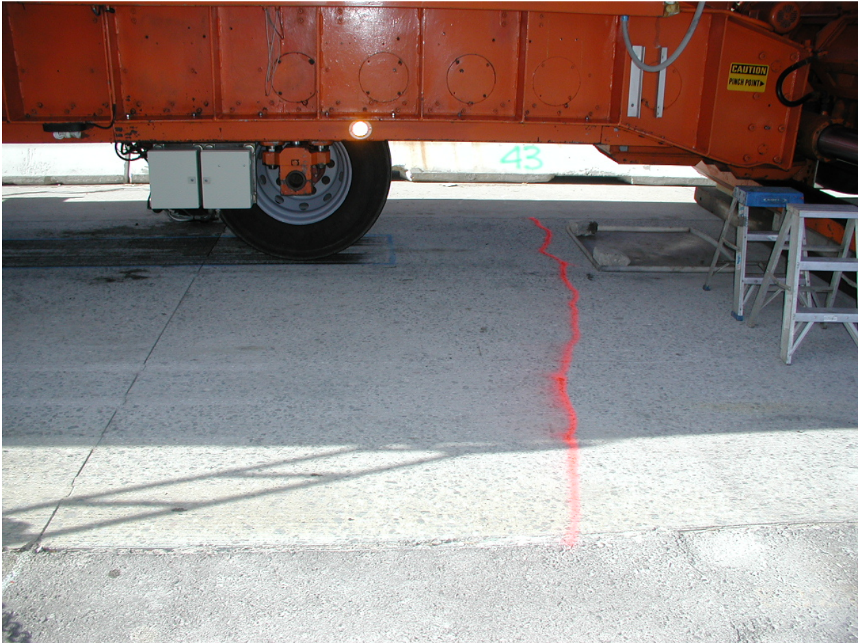
Figure 6.51. Slab 43 near Joint 42 on HVS Test Section 558FD after 2.002 million repetitions.
