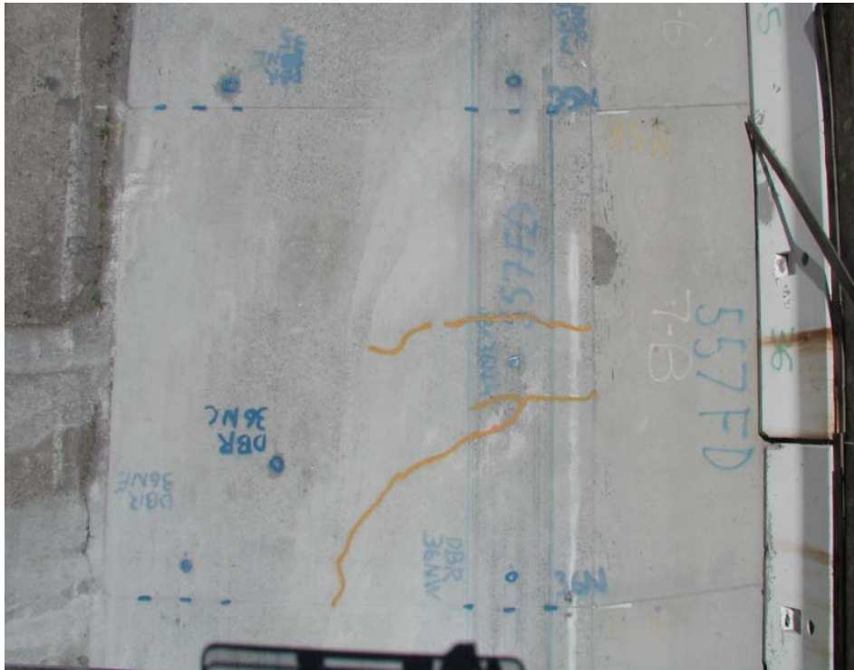
Appendix B. Figure 5. Slab 36 after DBR and HVS testing.
