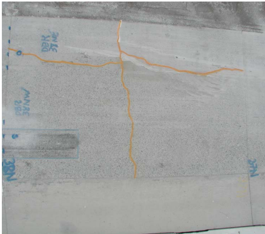
Appendix B. Figure 7. Slab 38 after DBR and HVS testing.
