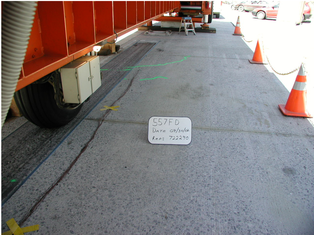
Figure 6.47. Mid-slab transverse cracking in Slab 36 after 722,290 repetitions.
