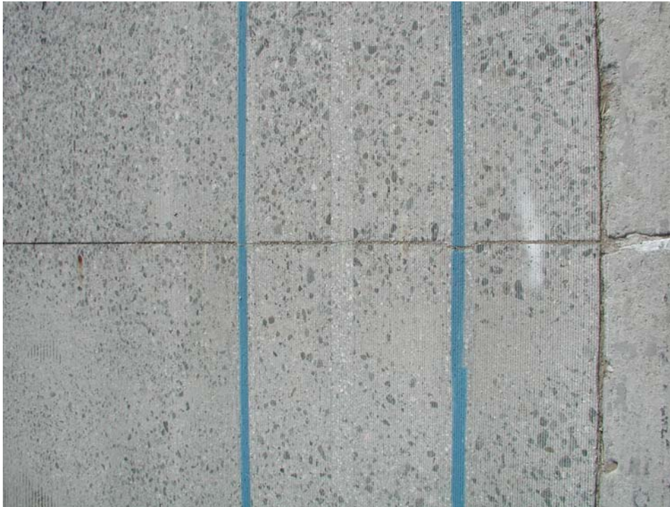
Figure 2.26. Close-up of surface texture of Section 557FD after dowel bar retrofit and grinding, and before HVS testing (blue lines painted on surface indicate future HVS wheeltrack).
