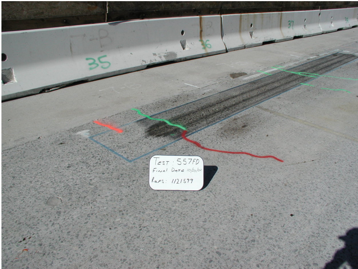
Figure 6.49. Final condition of Section 557FD after 1.122 million repetitions.
