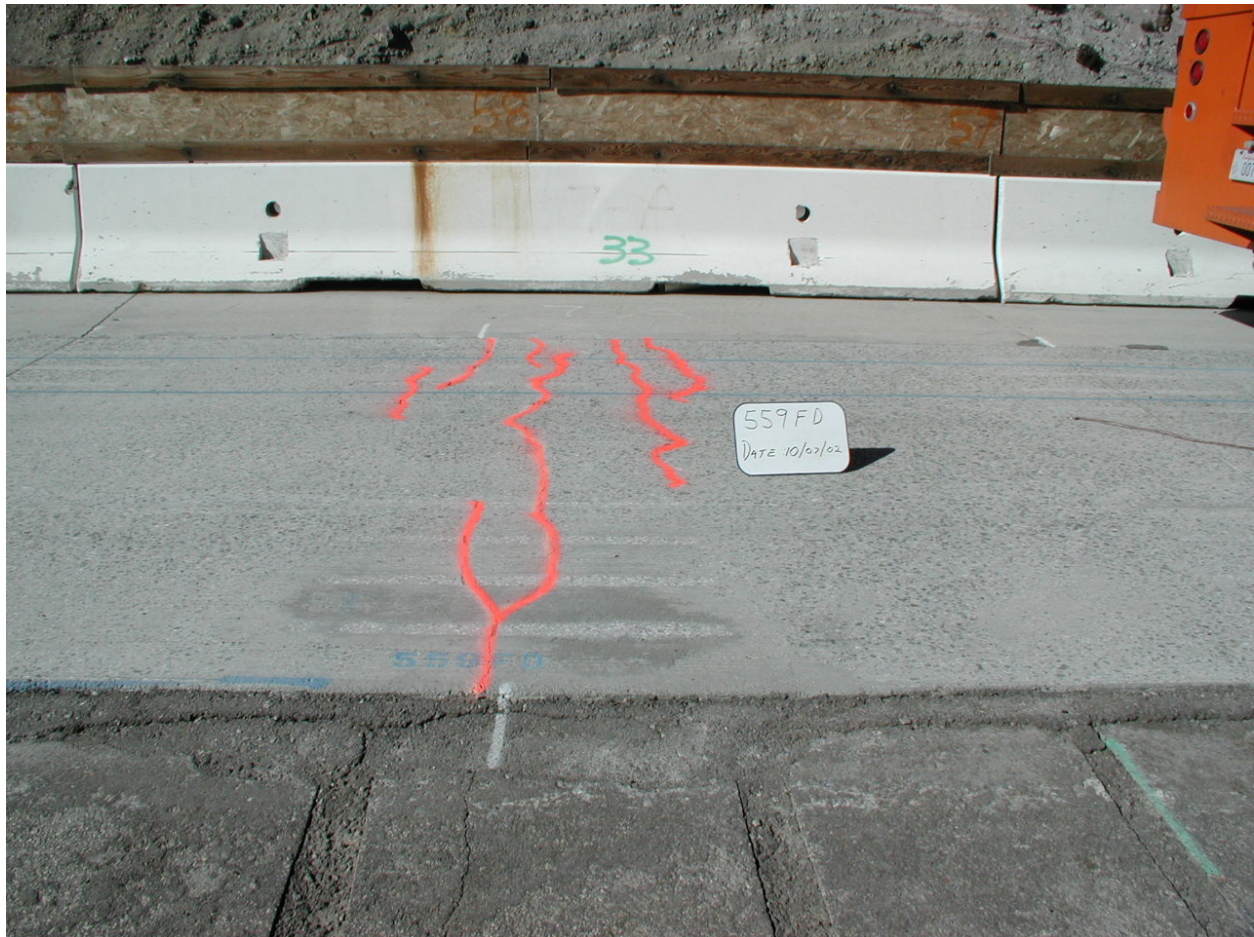
Figure 6.96. Final condition of Slab 33 showing additional cracking around Crack 1 after 2.001 million repetitions.
