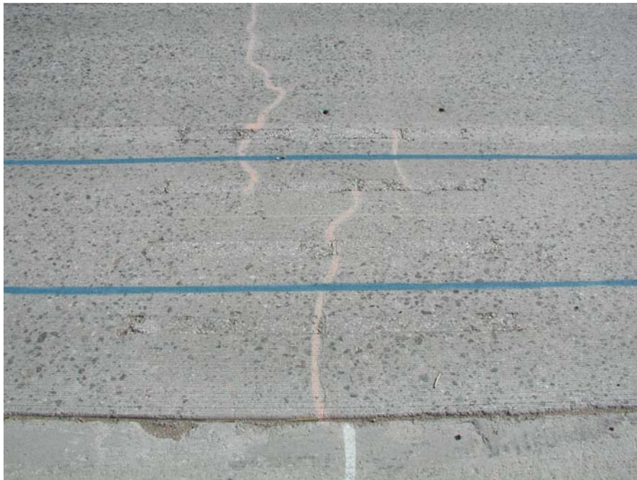
Figure 6.78. HVS Test Section 559FD, Crack 1, prior to HVS testing.
