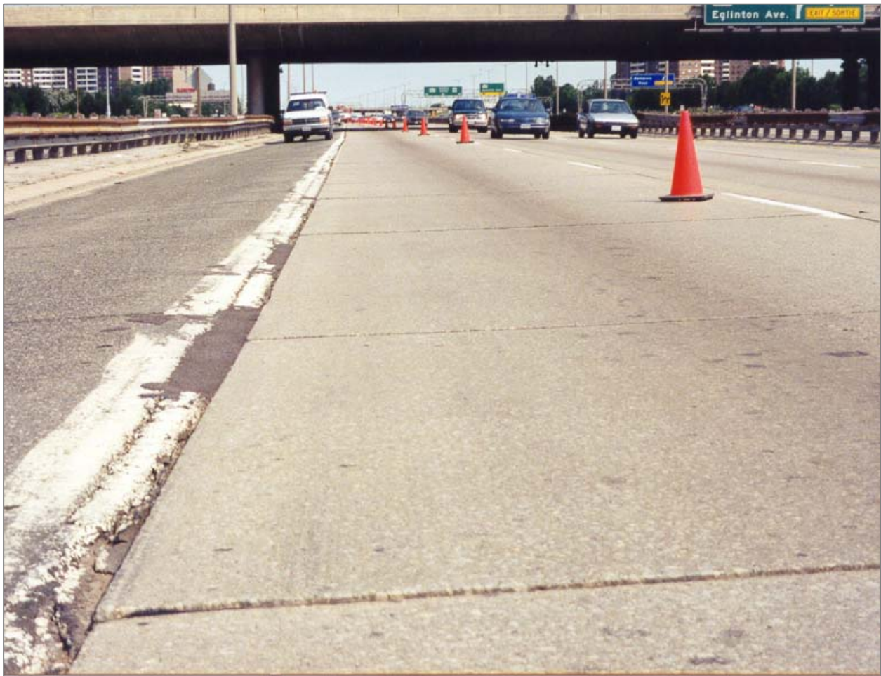
Figure 1.1. Upstream view showing faulting on an undoweled concrete pavement (courtesy of L. Khazanovich).
