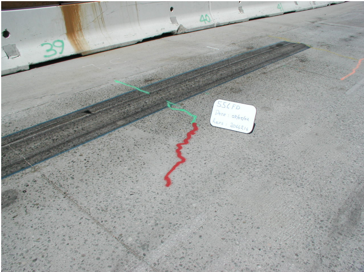
Figure 6.24. Cracking in Slab 39 after 2.066 million repetitions.
