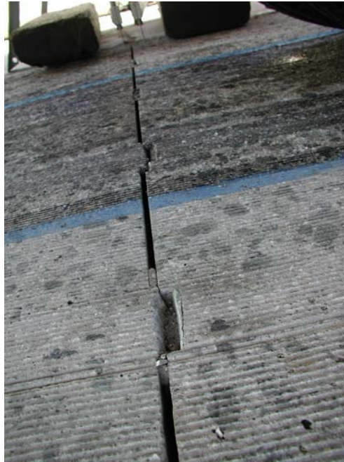
Figure 6.52. HVS Test Section 558FD, Joint 42 after 2.002 million repetitions.
