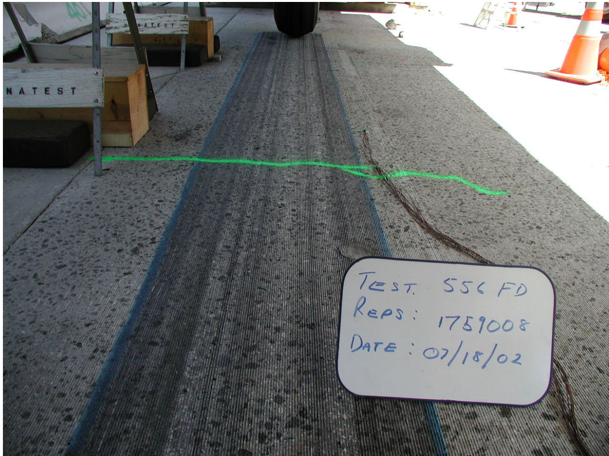
Figure 6.23. Cracking in the center slab (Slab 39) after 1.759 million repetitions.
