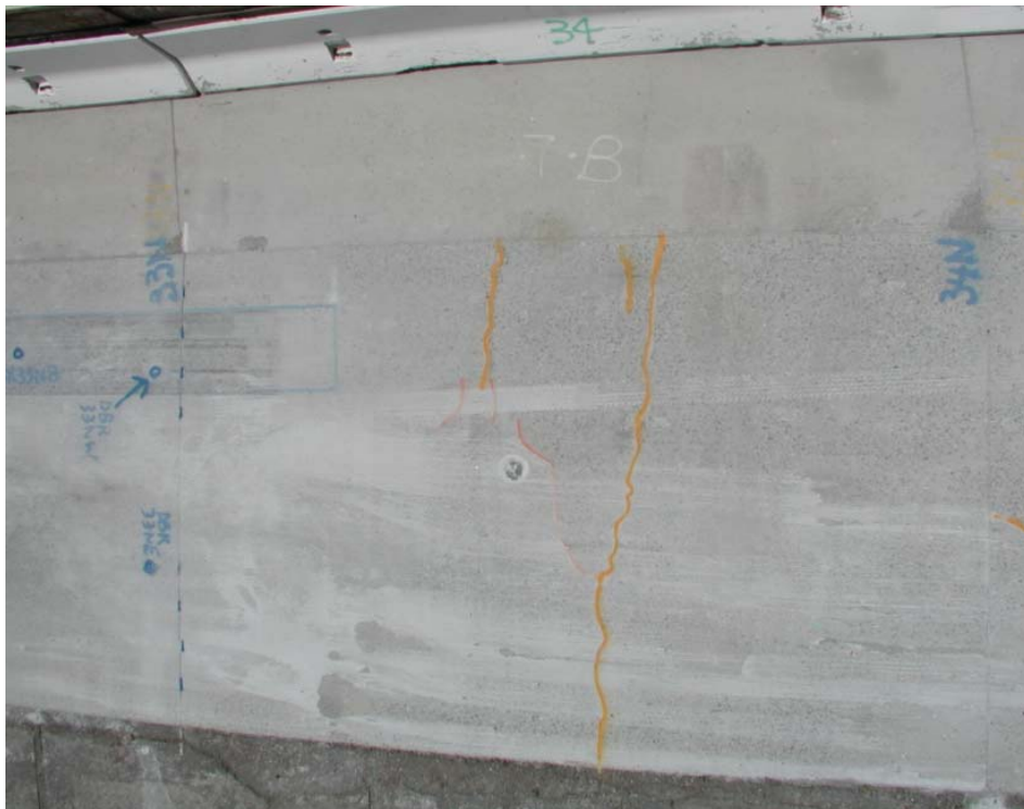
Appendix B. Figure 3. Slab 34 after DBR and HVS testing.
