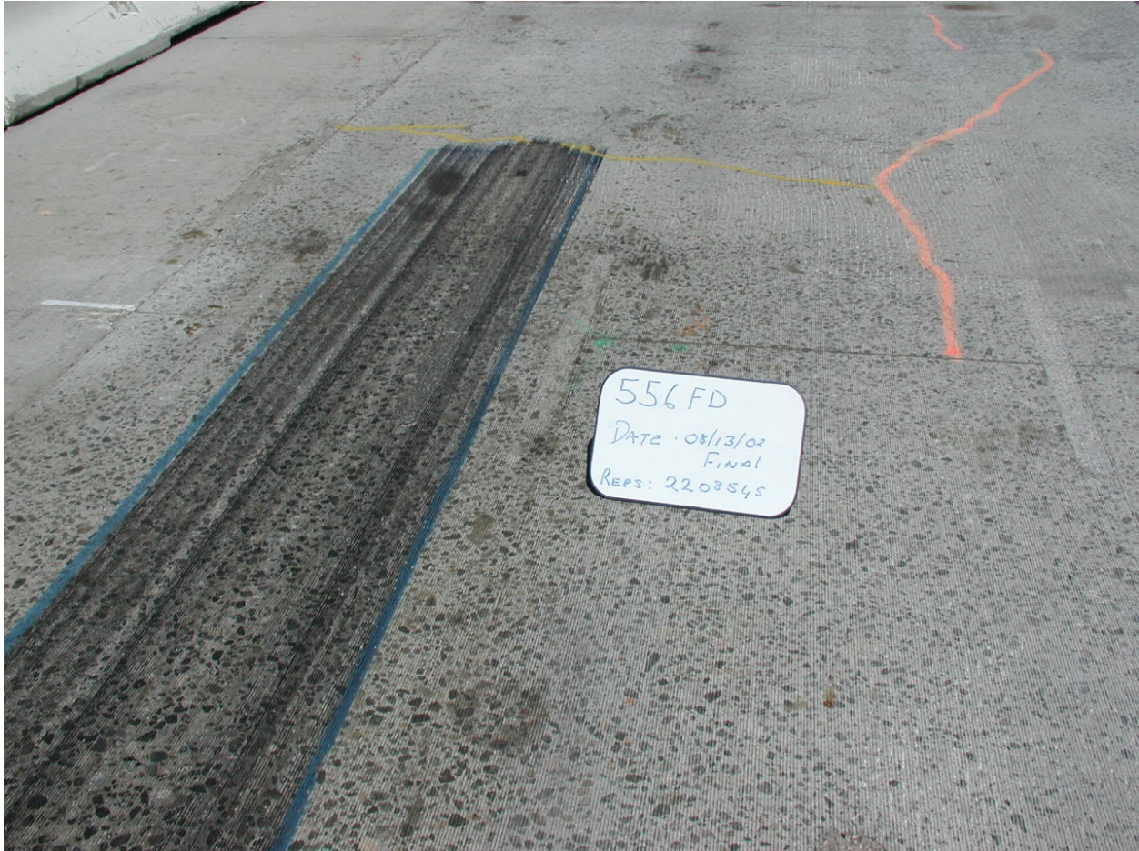
Figure 6.26. Close-up of Joint 39 at end of HVS loading after 2.209 million repetitions.
