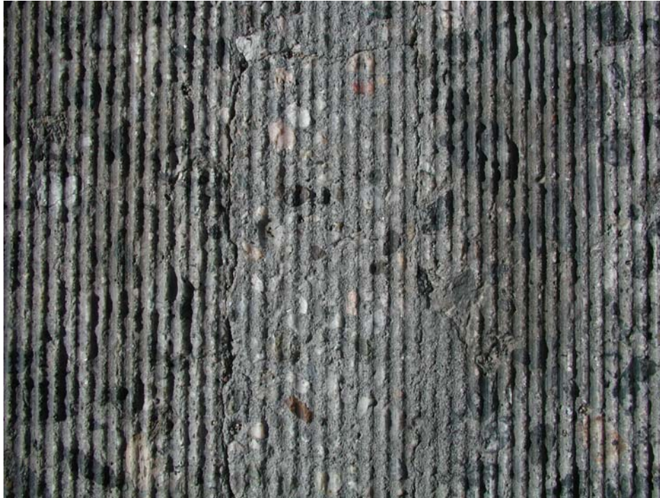
Figure 2.39. Photograph of DBR slot, Section 559FD, Slab 39, in June 2002, showing some separation of grout and slab.
