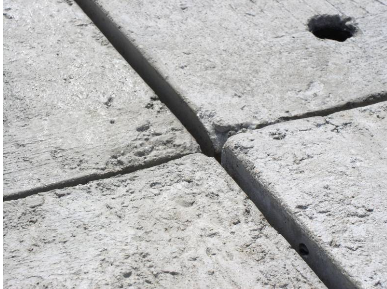
Figure 10. Misalignment of adjacent slabs causing surface irregularities.
