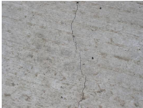
Figure 104. Part of a nontraffic-related transverse crack noticed on both sections after completion of the ungrouted tests.
