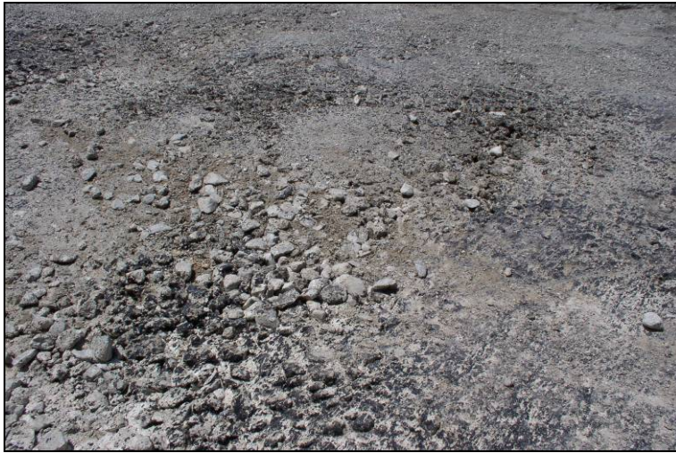
Figure 3. Texture of the completed CTB prior to construction of the Super-Slab® System.
