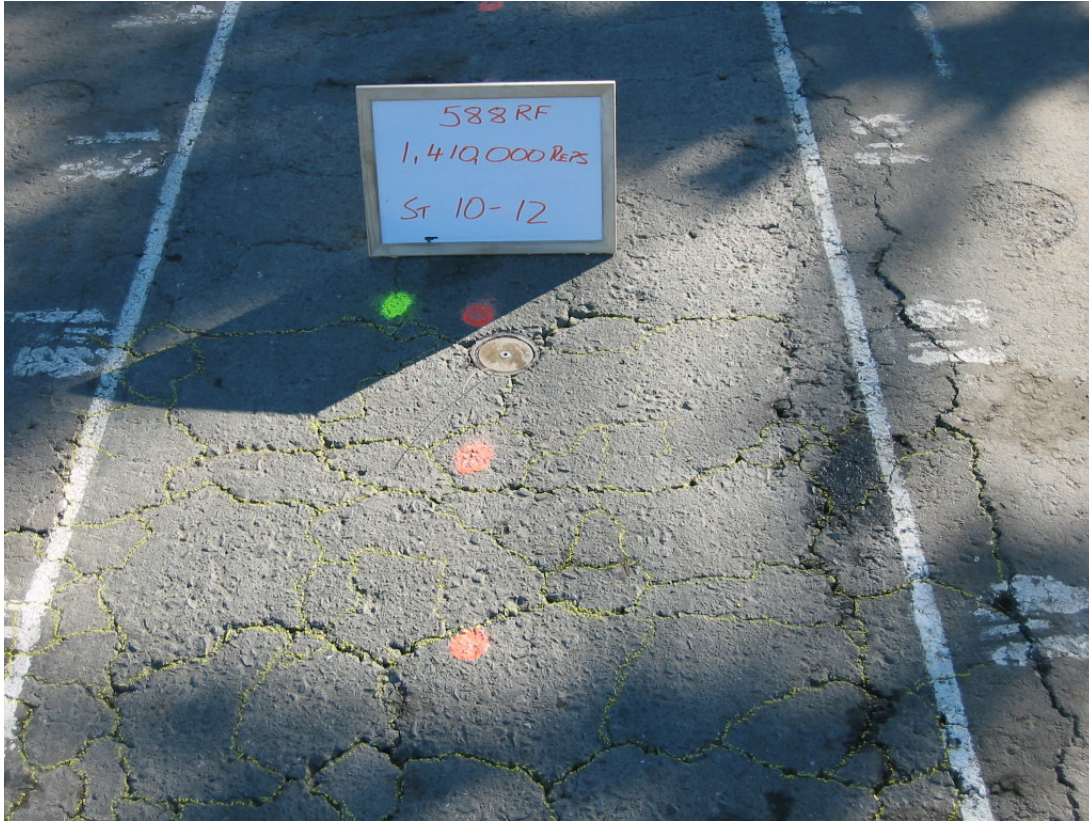
Figure 3.28: Surface cracks marked with crayon between Stations 10 and 12 at end of test.
