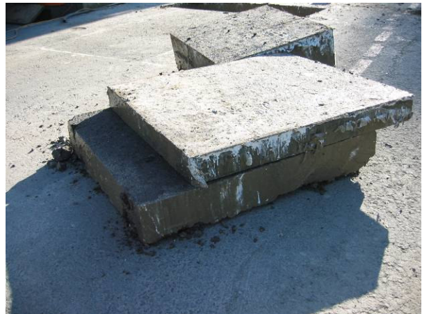
Figure 3.45: 588RF debonding between overlay and underlying layer.
