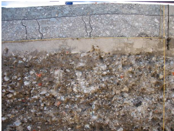
Figure 3.38: 587RF#4 cracks in underlying DGAC.
