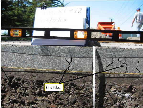
Figure 3.32: 586RF cracks in underlying DGAC.
