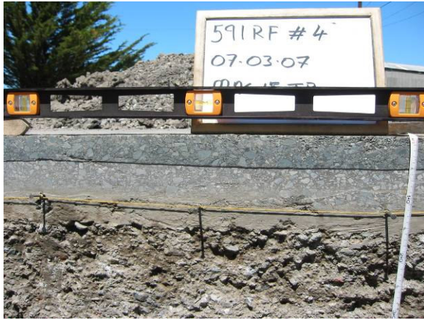
Figure 3.64: 591RF#4 rutting from Phase 1 trafficking.
