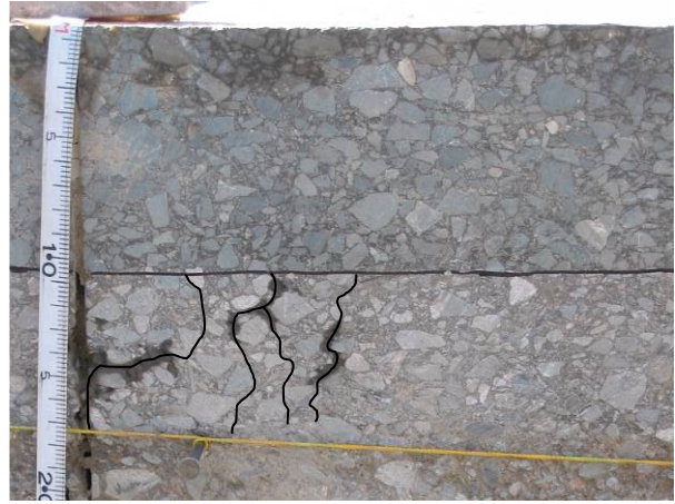
Figure 3.59: 590RF cracks in DGAC layer.
