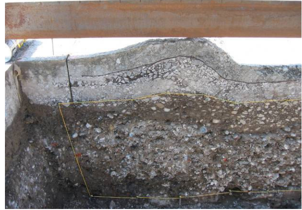
Figure 3.53: 589RF#12 severe displacement on edge of rut.
