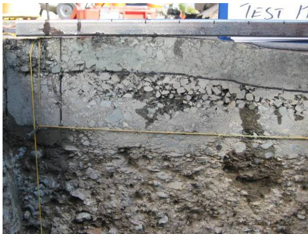
Figure 3.10: 581RF segregation in DGAC layer.
