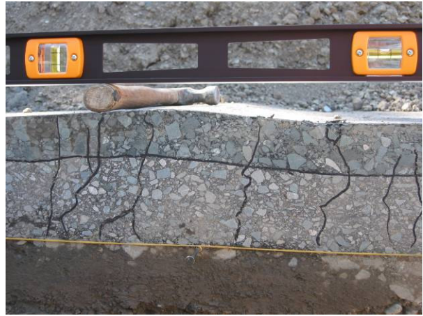
Figure 3.37: 587RF#4 cracks in overlay and underlying DGAC.
