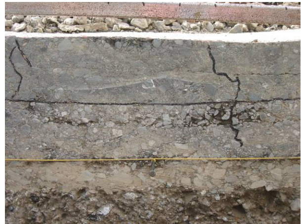
Figure 3.47: 588RF cracks in overlay and underlying DGAC.
