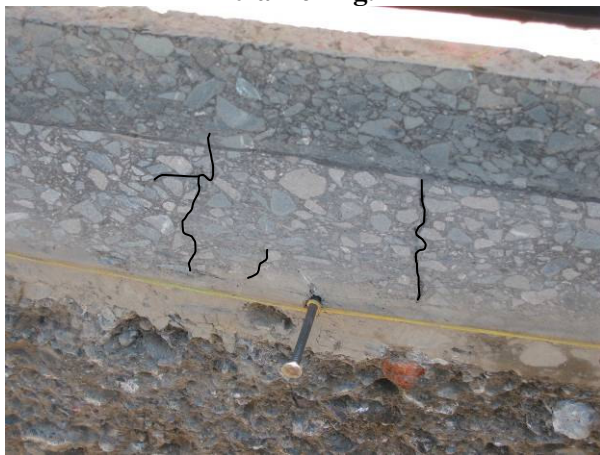
Figure 3.66: 591RF cracks in underlying DGAC.
