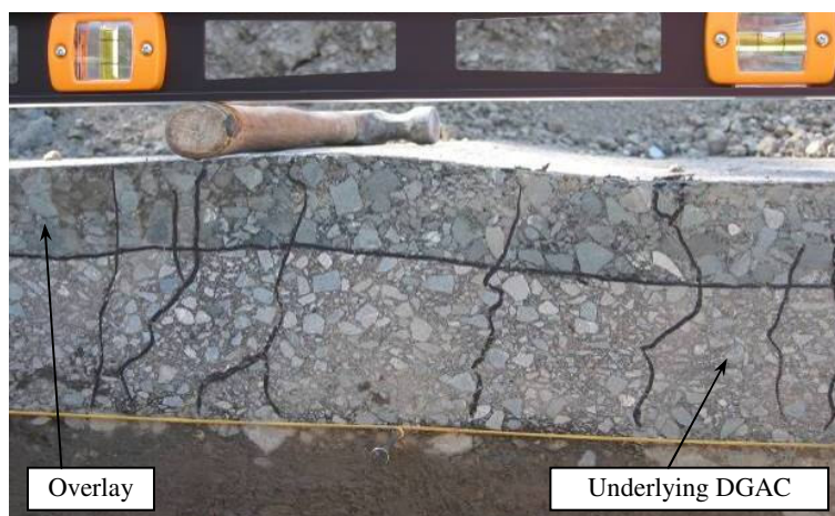
Figure 4.10: Test pit profile showing highlighted cracks (RAC-G section).
