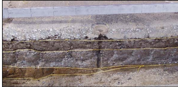
Figure 4.31: Test pit on Section 595FD after HVS trafficking.
