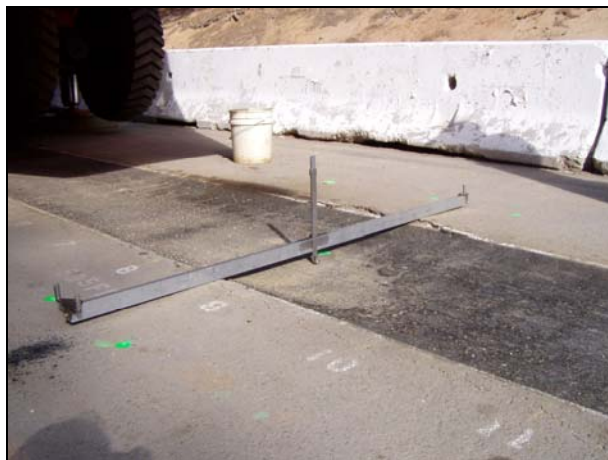
(a) Rut on Section 595FD at end of test
