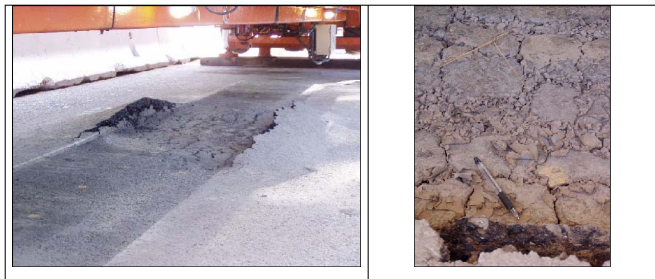
(a) Shear failure between Stations 7 and 8
