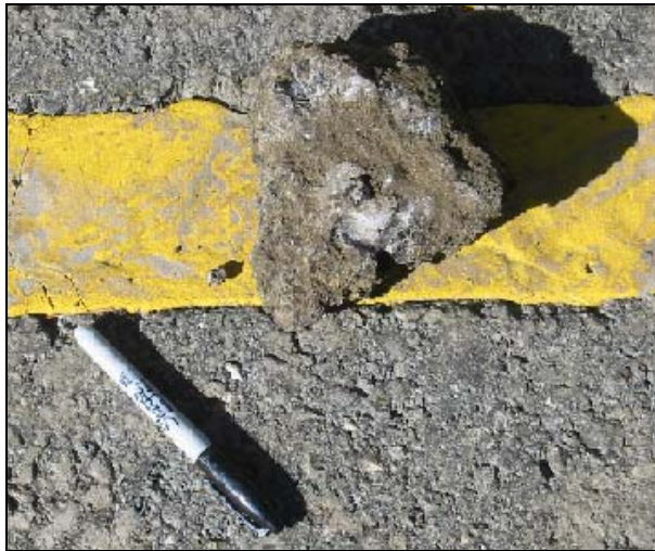
Figure 4.20: Intact piece of reclaimed asphalt concrete found in the mainline test pit.
