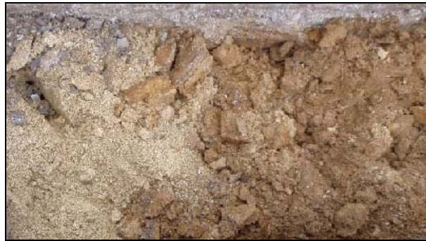
Figure 4.32: Two materials in subgrade on Section 595FD.
