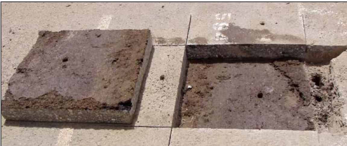
Figure 4.27: Bond between asphalt concrete surfacing and the treated base on Section 594FD.
