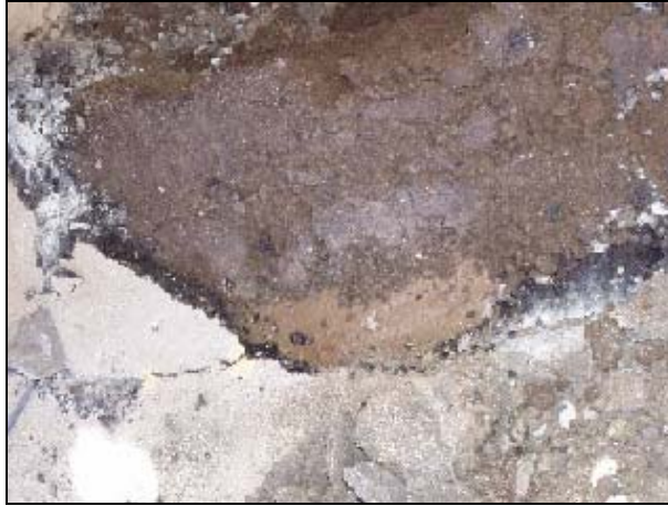
Figure 4.34: Mud between the AC surfacing and treated base, on the side of Section 596FD.
