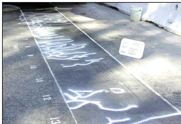
Figure 5.17: Visual condition of Section 594FD at the end of the test.
