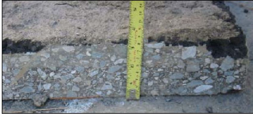
Figure 4.22: Good bond between asphalt concrete and foam asphalt base layer on Section 593FD.
