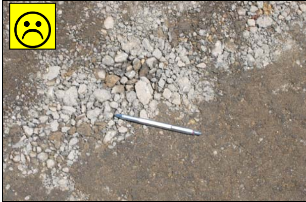
Figure 6.44: Segregation after grading.
