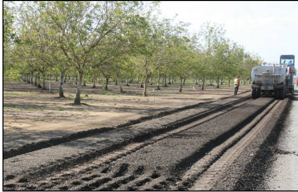
Figure 6.34: Differential compaction in recycling train wheelpaths.
