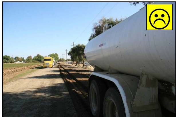
Figure 6.40: Primary compactor too far behind recycling train.
