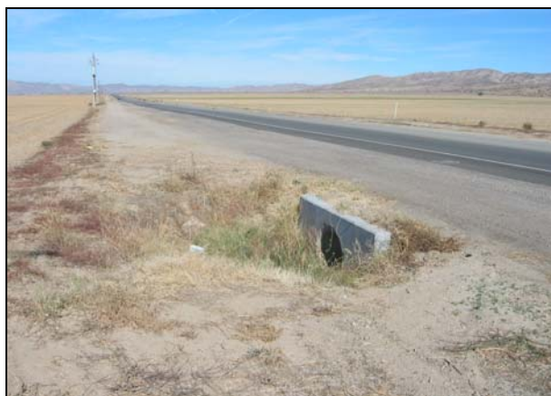
Figure 2.4: Blocked side drain and culvert.
