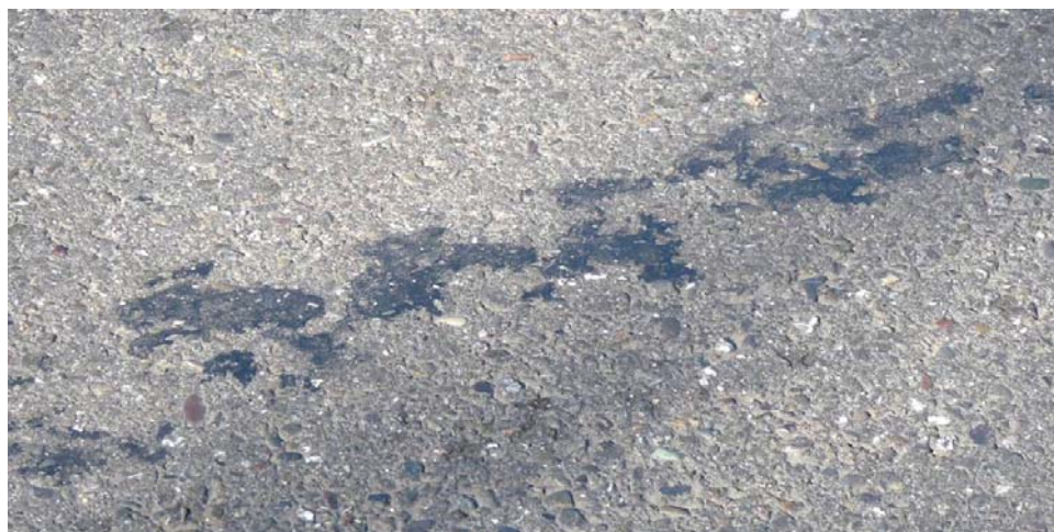
Figure 1.13. Bleeding where bitumen covers part of the pavement surface.
