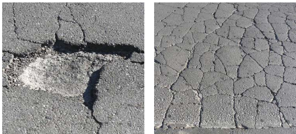
Figure 1.12. Pothole (to the left) and alligator cracking (to the right).
