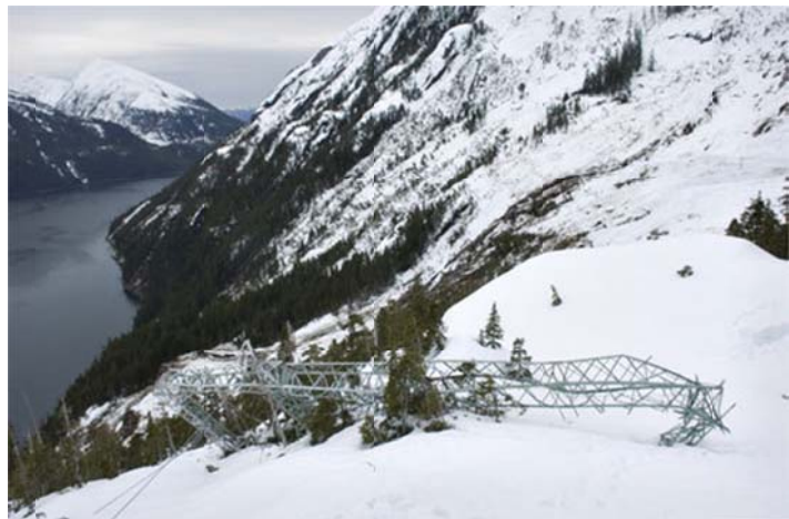
Figure 2: Tower on the Snettisham transmission line destroyed by an avalanche (Michael Penn, Juneau Empire).
