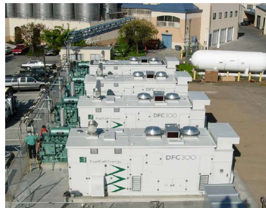
Four 250 kW molten carbonate fuel cells power the Sierra Nevada Brewery
