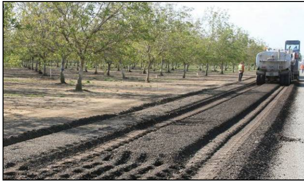
Figure 7.8: Differential compaction in rotary mixer/recycling train wheelpaths.
