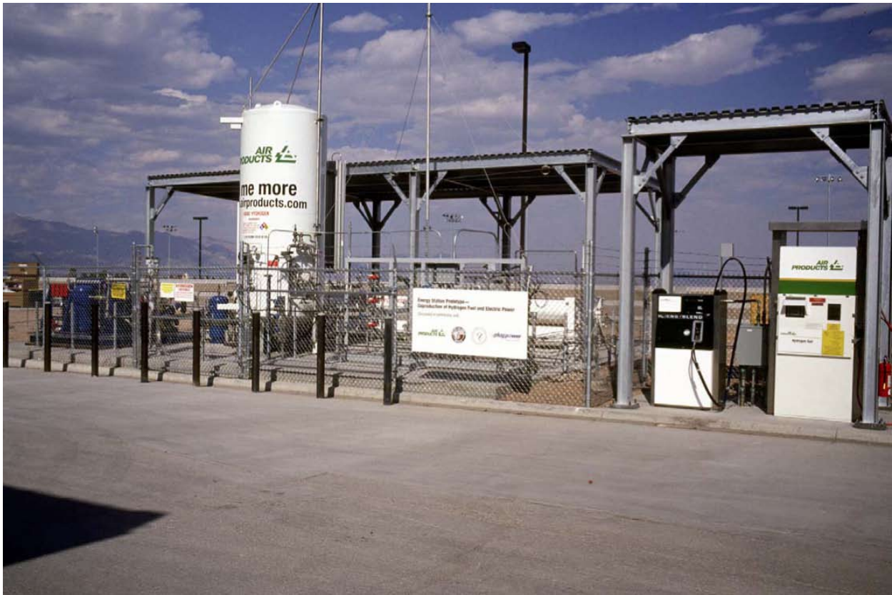
Figure 3: The Las Vegas Energy Station
