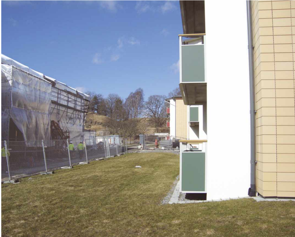
Figure 5. Renovation of a neighbourhood. Residents live on site during renovations, but there is a good atmosphere on the work site. Source: Carley Friesen.
