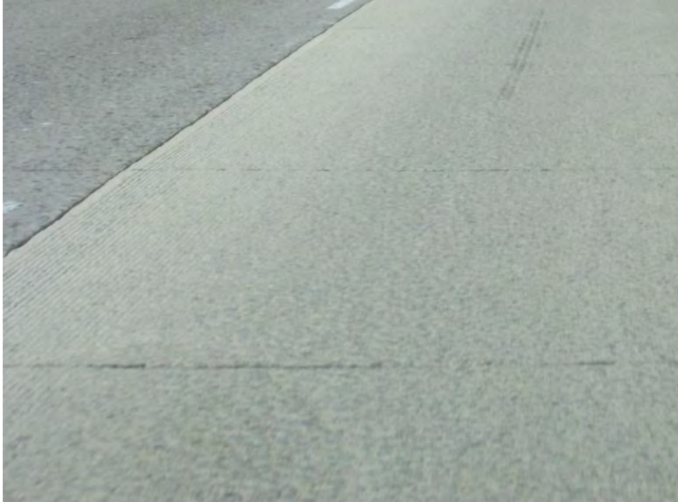
Figure C.2: Evidence of original longitudinal tines outside of the wheelpaths of Section QP-142.2 after one year of traffic.
