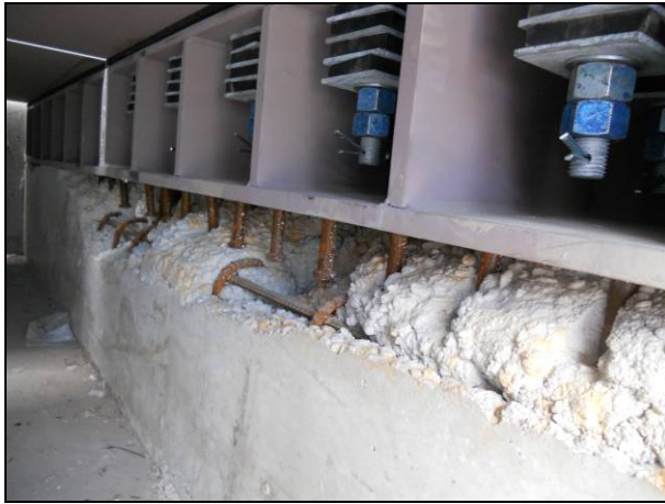
Figure 2.10: Concrete pour problem on channel assembly structure.
