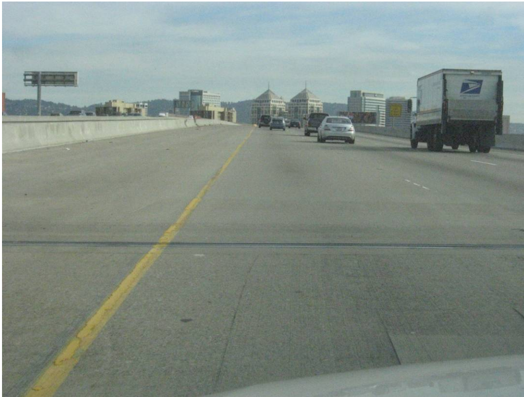
Figure 4.27: Surface and first measured joint on Section QP-121.1.
