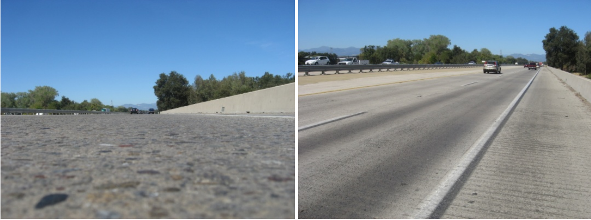
Figure 4.76: Close up view of wheelpath texture in the wheelpaths and overall view of Section QP-141.1.
