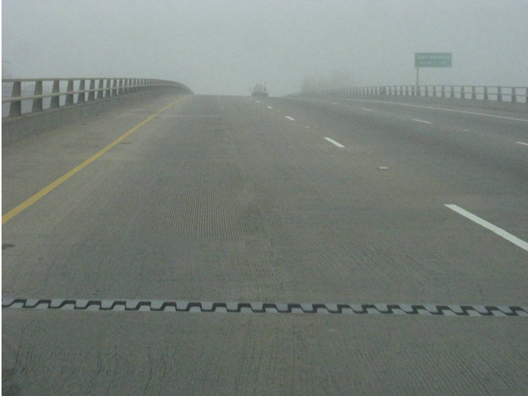
Figure 4.120: Surface and special longer span joints (one of four) on Section QP-151.1.
