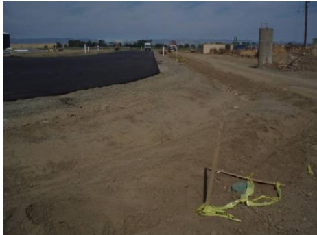
June 30, 2008- Northern edge, facing west; Pavement layer added to gravel material and shaping of road-side verge and swale
