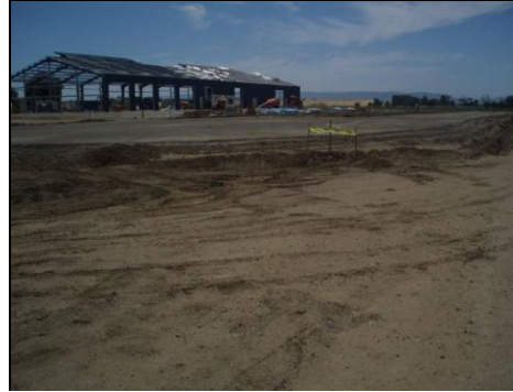
June 20, 2008- Northern edge, facing west; Resurfacing and compacting of gravel material on test track
