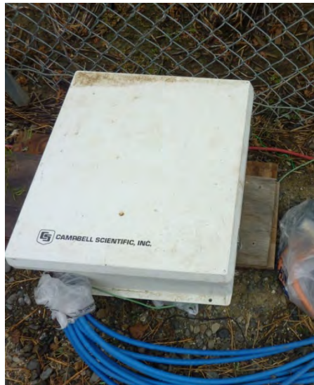
(c) Data collection system (outside)
