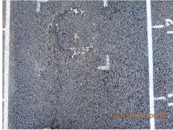
(b) Damage caused by the use of Ecoflex sealant
