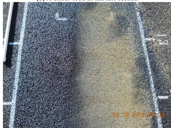
(d) Signs of subgrade rutting and crack initiation near Station 13 but no moisture damage in the asphalt
