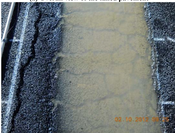
(c) Severe cracking and punch down near Station 7
