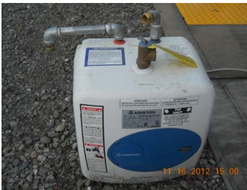
(a) Water heater
