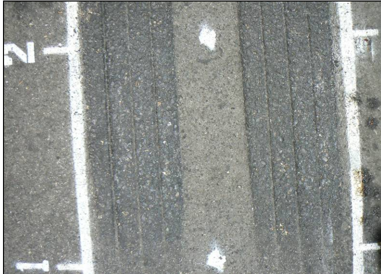
Figure 4.29: 622HA: Section photograph at test completion.
