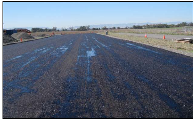
Figure 2.25: Differential penetration of prime coat.
