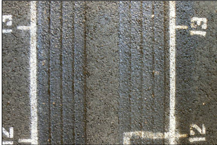
Figure 4.20: 621HA: Section photograph at test completion.
