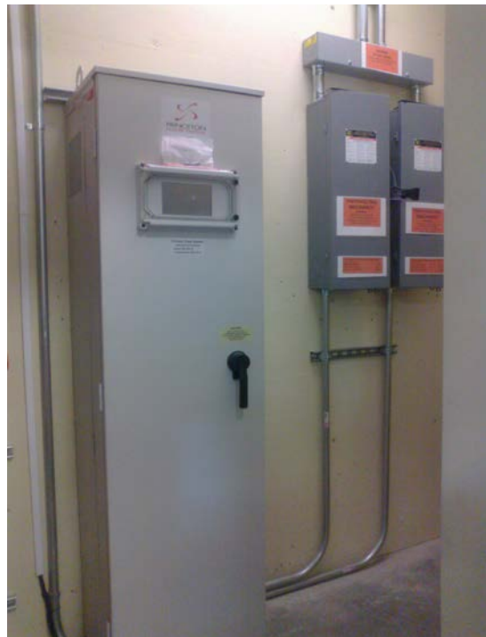
Figure 14: Bi-directional Inverter and Disconnect & Bypass Switches
