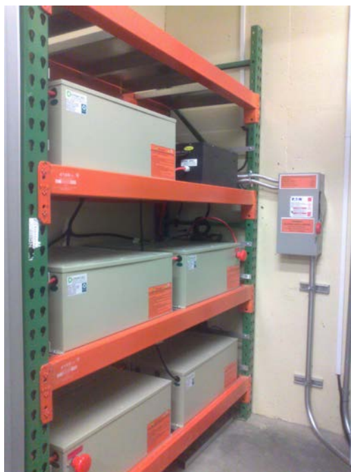
Figure 13: Battery Bank and Battery Management System
