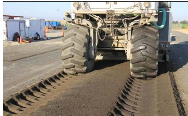
Figure 3.15: FDR-EE: Inconsistent emulsion application across width of test track.
