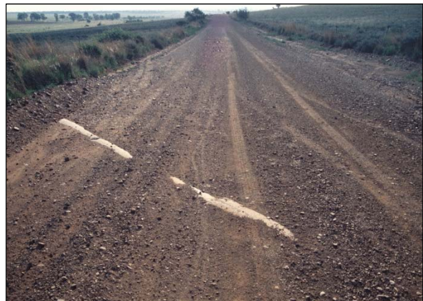
Figure B.2: Poor gravel road.
