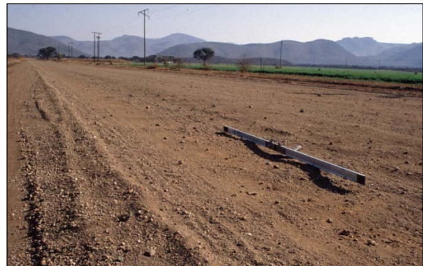
Figure B.12: Washboarding and raveling.
