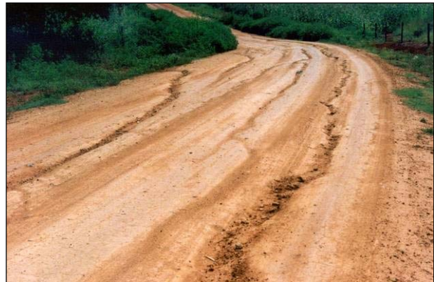
Figure B.9: Longitudinal erosion.
