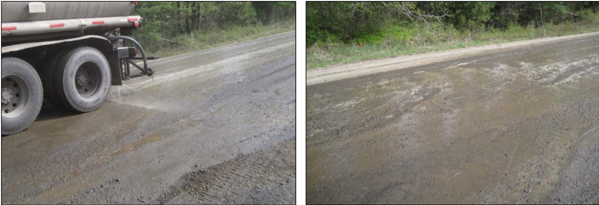
Figure 5.13: Overspray leading to ponding and runoff of treatment.
