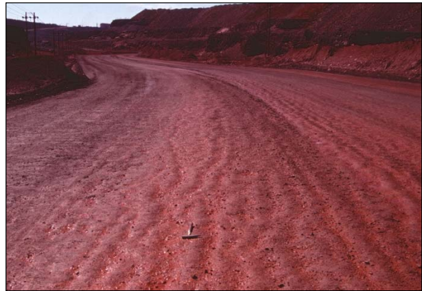
Figure 2.2: Erosion caused by repeated water spraying.
