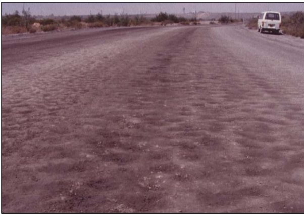
Figure 2.1: Potholes caused by repeated water spraying.
