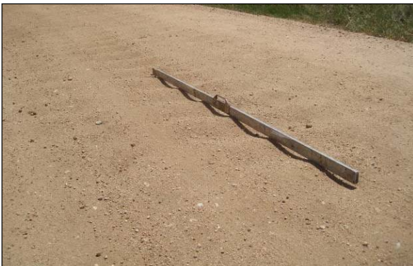
Figure B.11: Washboarding (corrugation).
