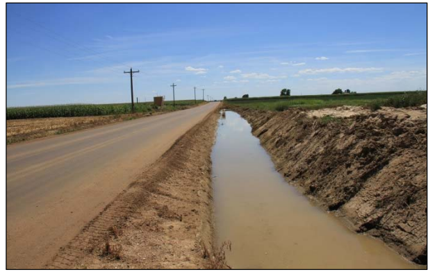
Figure 5.10: Water ponding next to road.
