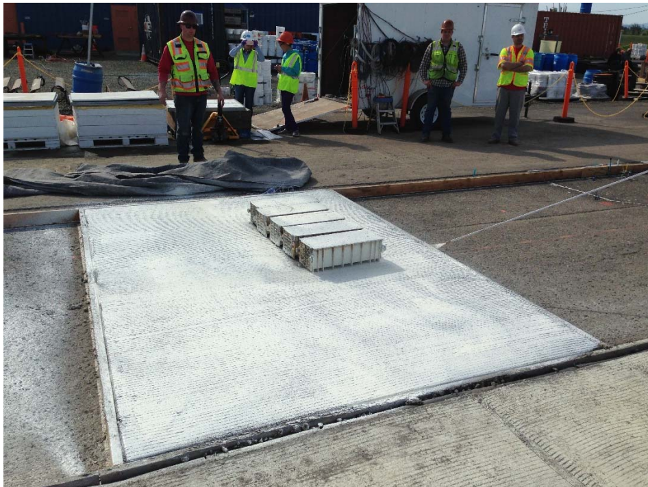
Figure A.92: Concrete beams ready to be cured on top of pavement slab (California Test 524).
