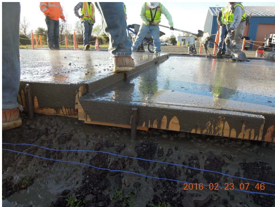
Figure A.40: The difference in PCC layer thickness between Section A (left, 150 mm [6 in.]) and Section B (right, 115 mm [4.5 in.]).
