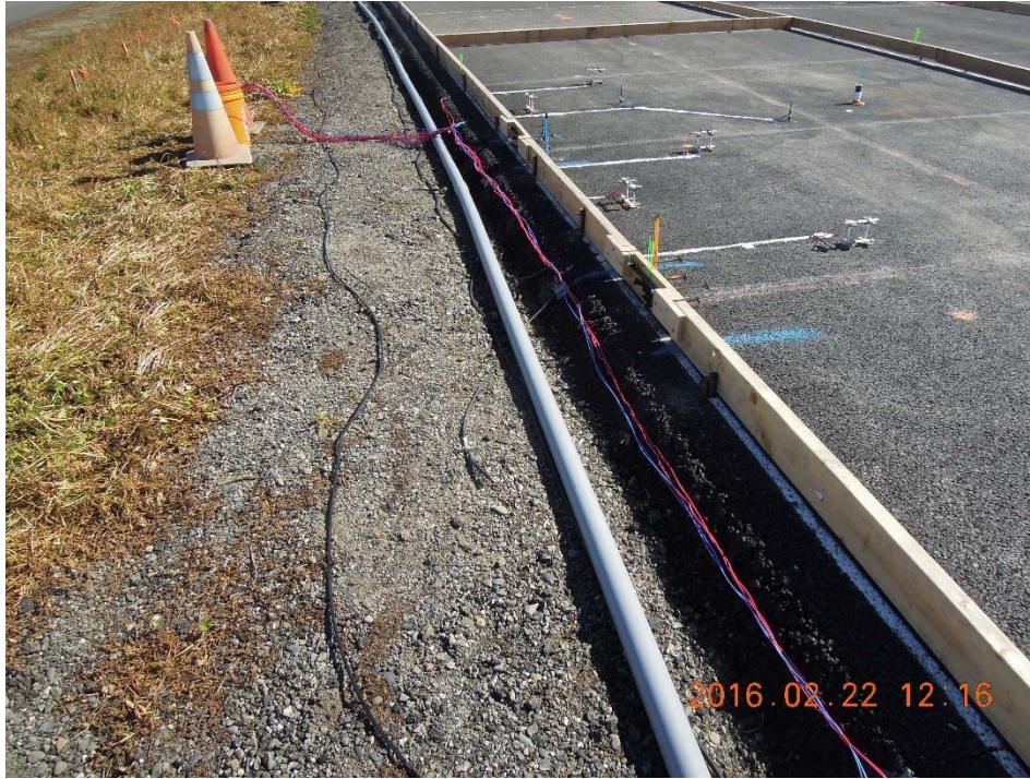
Figure A.23: Protective pipes for instrumentation wiring.
