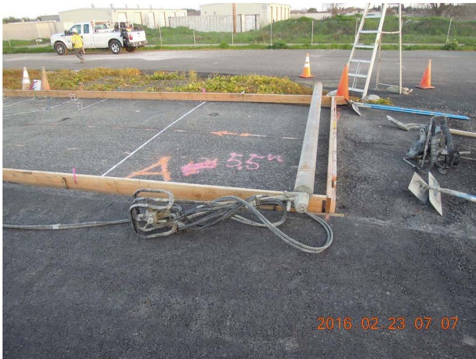
Figure A.30: Roller screed on Section A prior to arrival of concrete.
