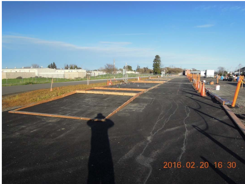
Figure A.13: Lane 1 with form work and instruments ready to be paved on new RHMA-G.
