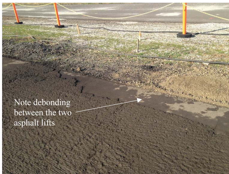
Figure 4.3: The appearance of the surface after milling shows debonding of the two older asphalt lifts.
