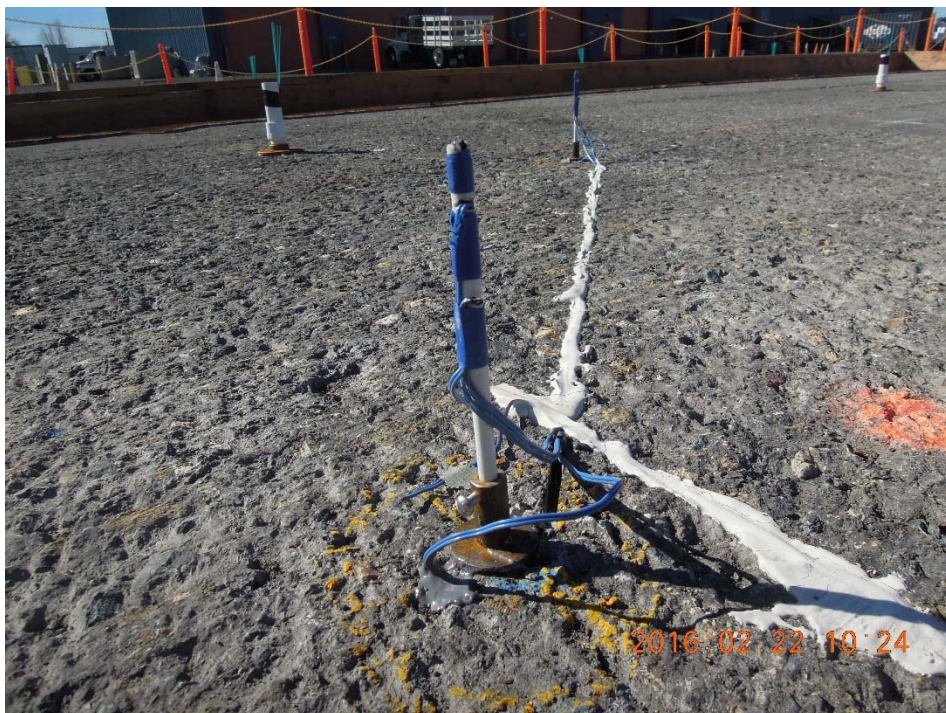
Figure A.20: Close-up of thermocouples attached to a fiberglass rod.
