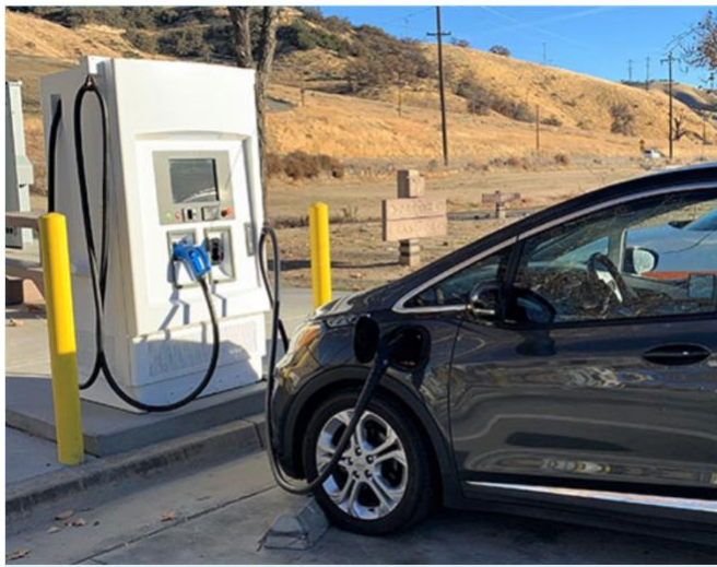
Four new EV fast chargers are located at Tejon Pass Rest Area.
