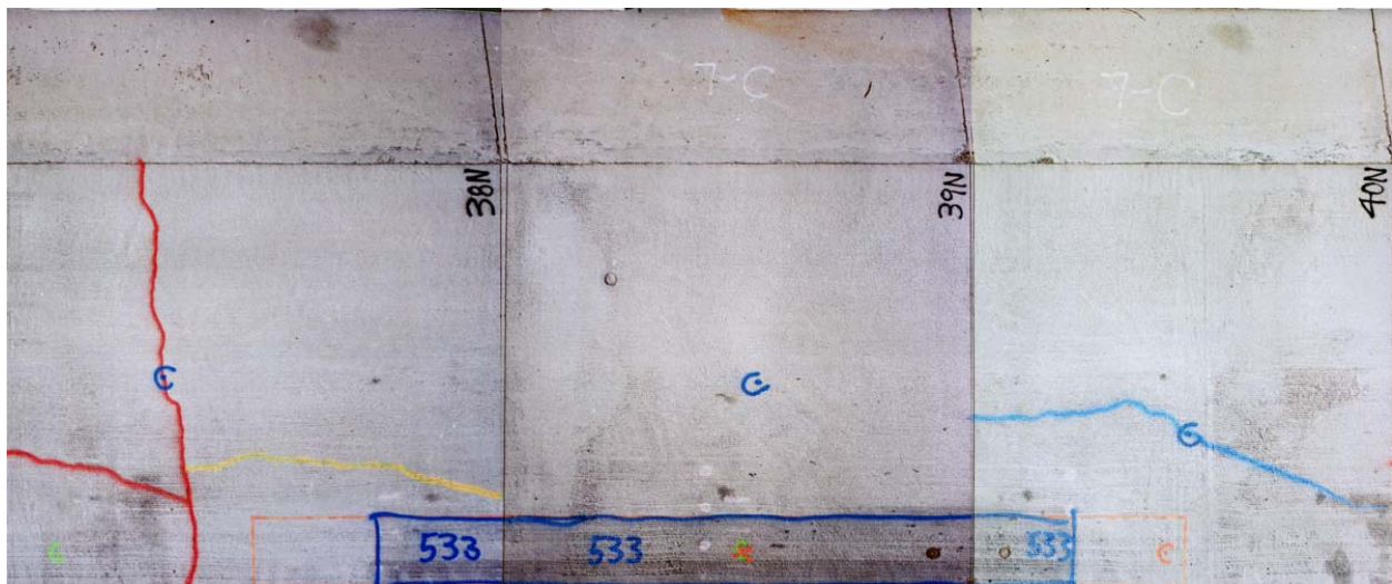
Figure 18. Composite image of Test 533FD showing cracks.
