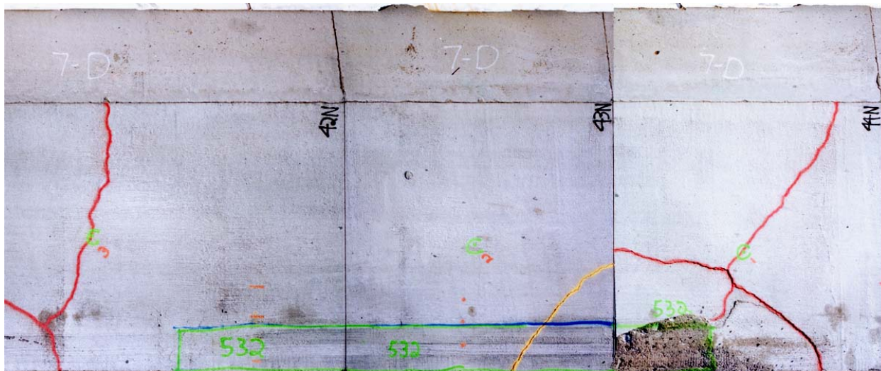
Figure 14. Composite image of Test 532FD showing cracks.
