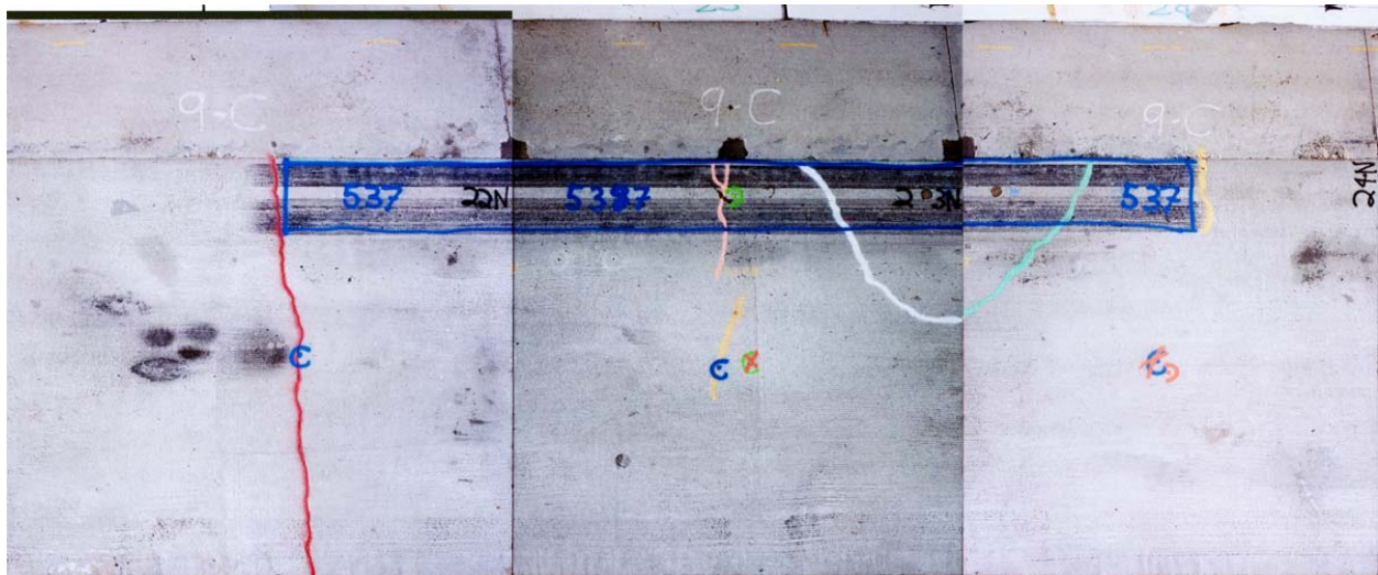
Figure 54. Composite image of Test 537FD showing cracks.
