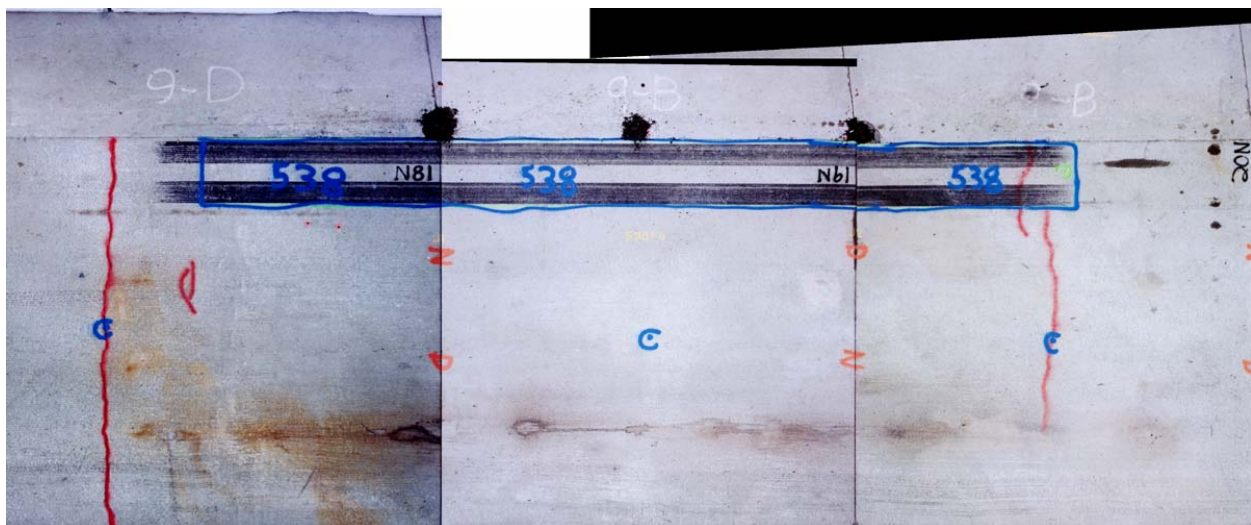
Figure 72. Composite image of Test 538FD showing cracks.
