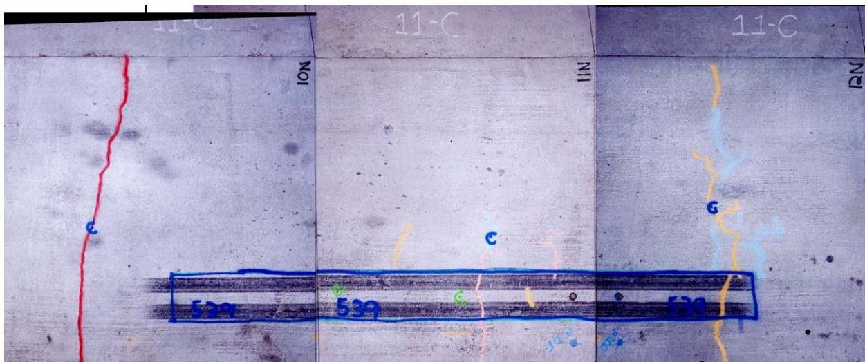
Figure 85. Composite image of Test 539FD showing cracks.
