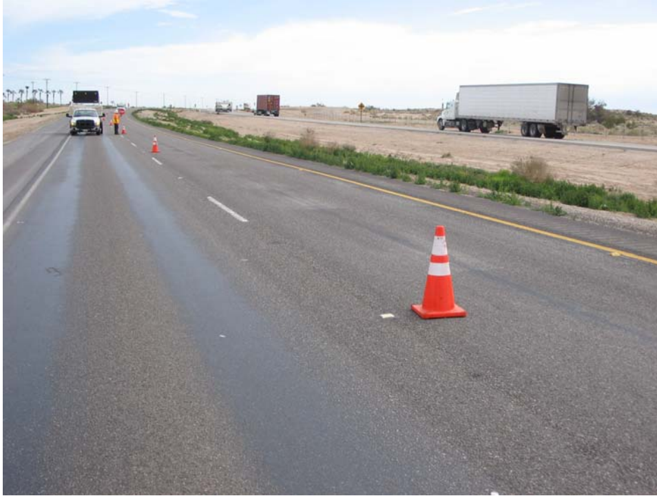
Figure 12. Station 652+40, facing south—flushing evident in #2 lane.
