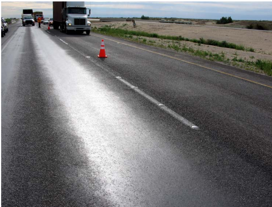
Figure 7. Station 610+40, facing south—flushing evident in #2 lane.
