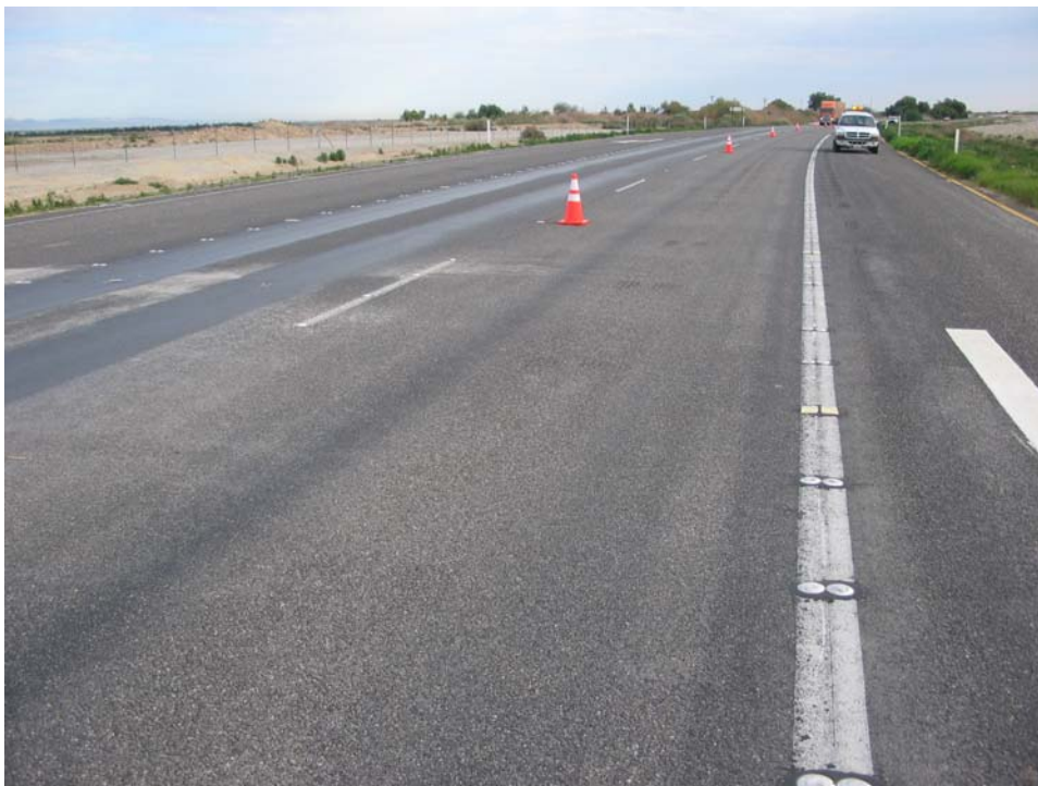
Figure 9. Station 616+37, facing south—note that #1 lane is clear of flushing and rutting while #2 lane shows clear evidence of flushing and rutting.
