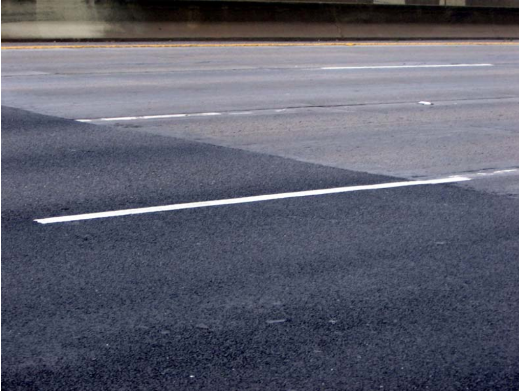
Figure 25. End of open graded section (northbound direction)
