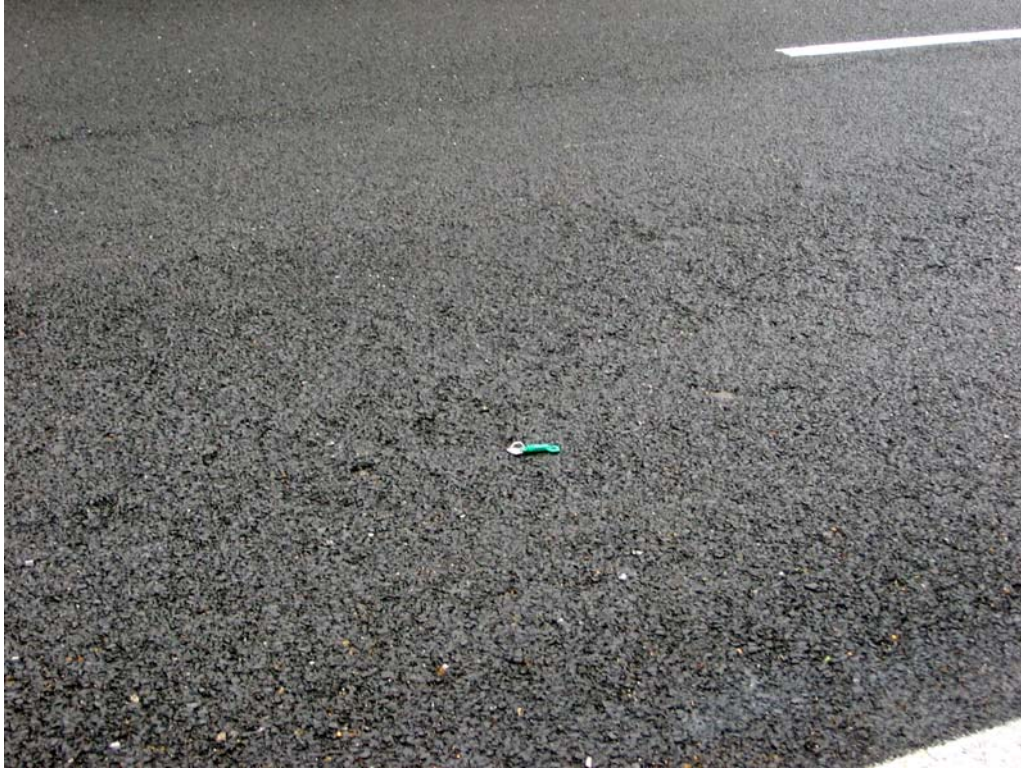
Figure 22. Raveling at Station 56+80 (northbound direction).
