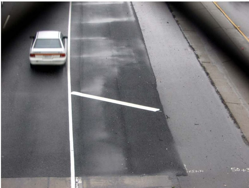
Figure 17. Ponding at Station 50+00 (outside lanes, northbound).
