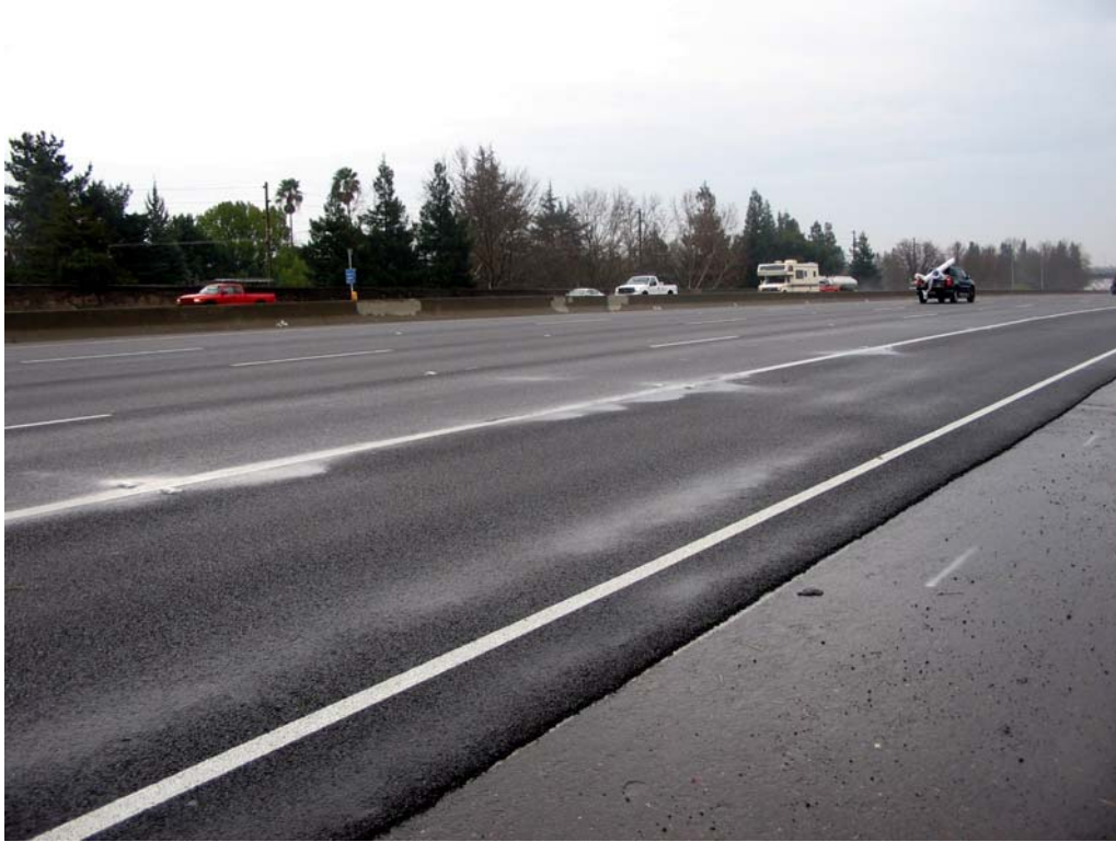
Figure 13. Polishing and mild rutting near Station 54+50 (outside lanes, southbound).
