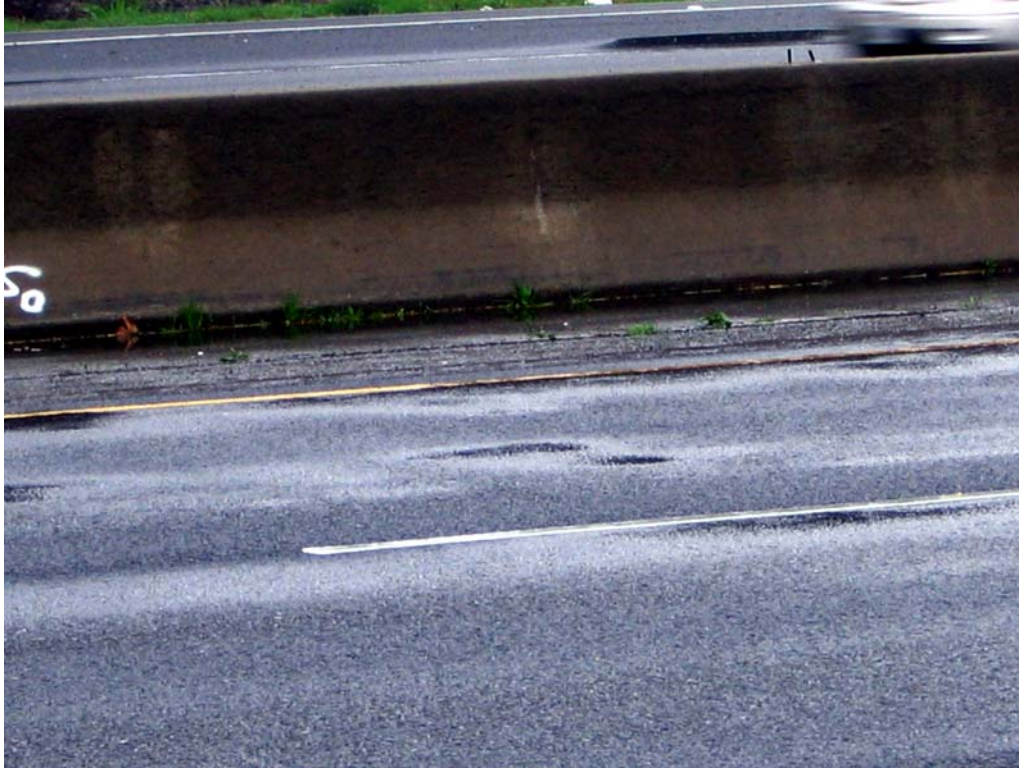
Figure 11. Ponding at Station 51+60 (inside lanes, southbound).
