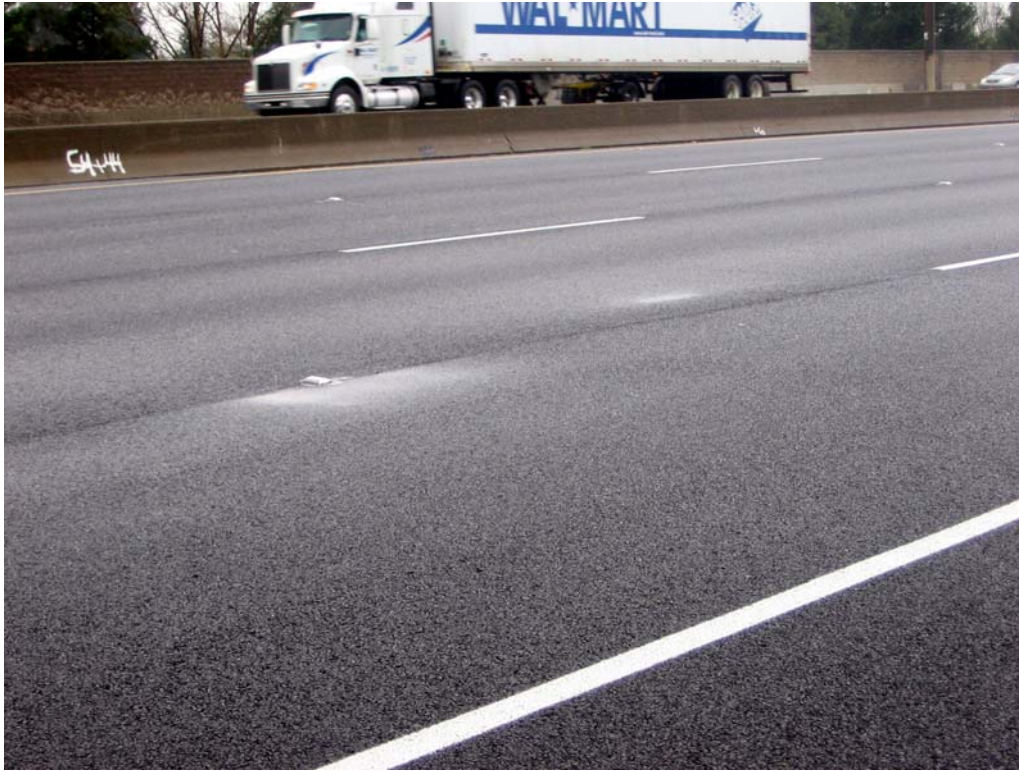
Figure 20. Ponding between at Station 54+44 (inside lanes, northbound).
