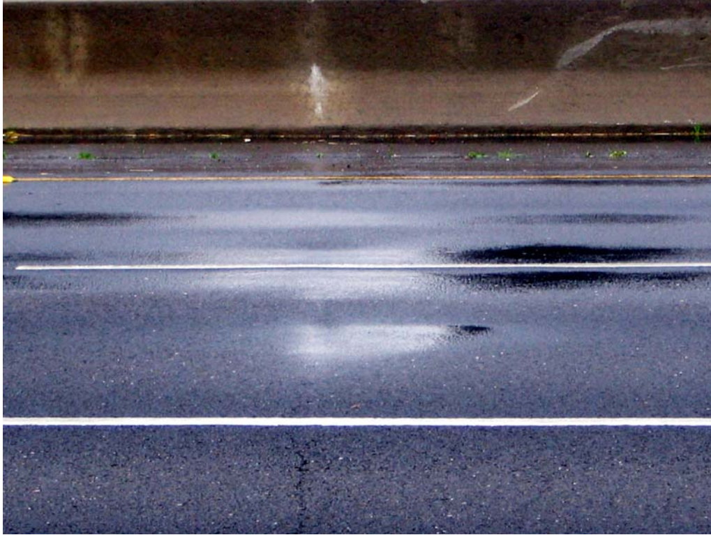
Figure 9. Ponding between Station 51+00 and Station 51+60 (inside lanes, southbound).
