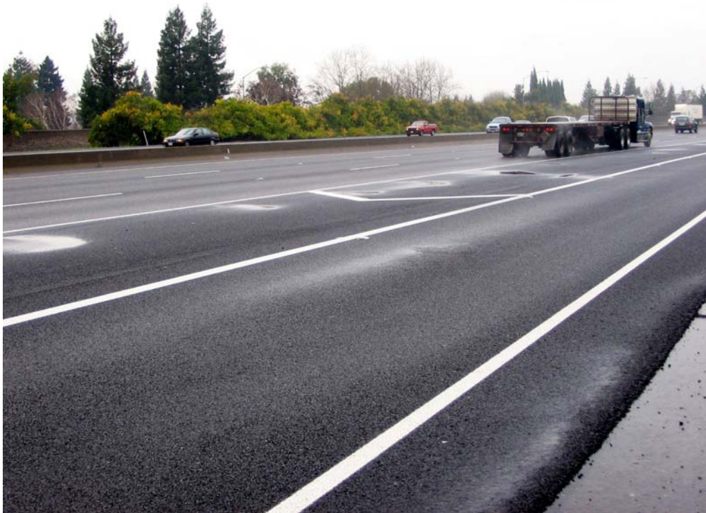
Figure 19. Ponding between Station 53+00 and Station 54+00 (outside lanes, northbound)
