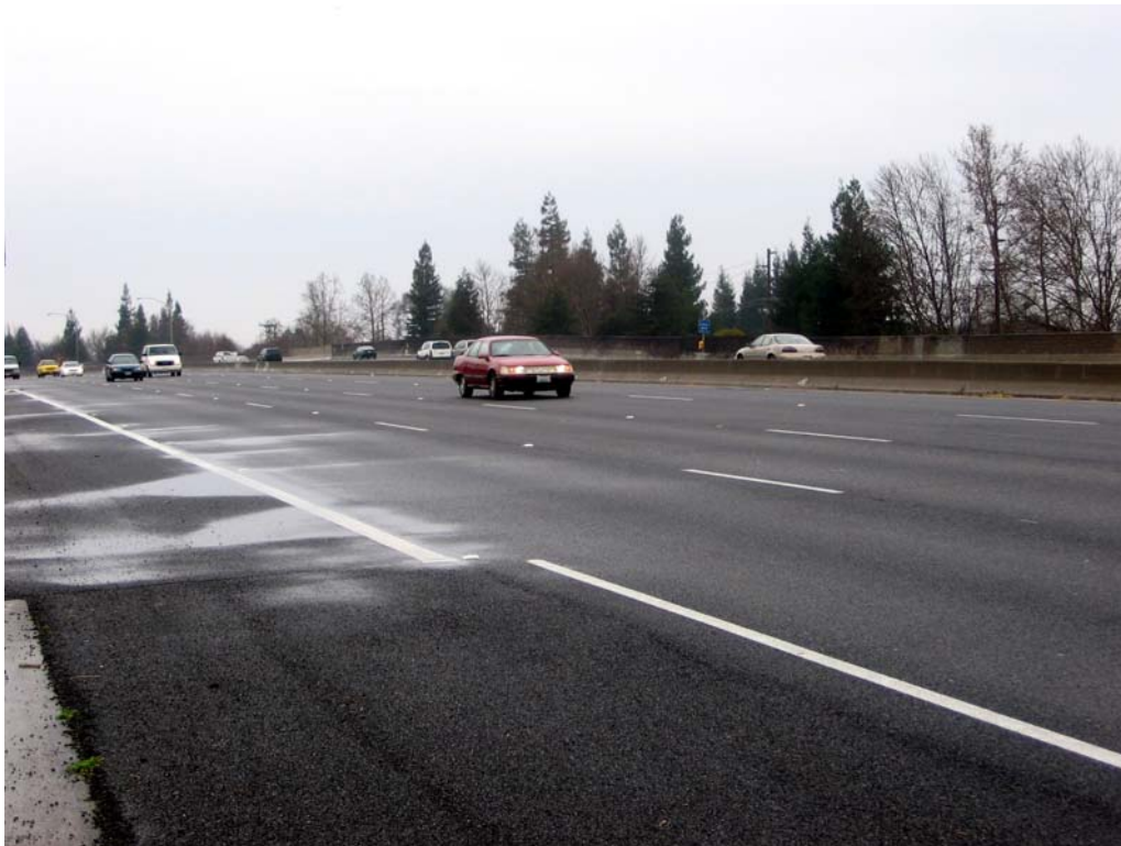
Figure 12. Ponding looking north from Station 55+00 (outside lanes, southbound).
