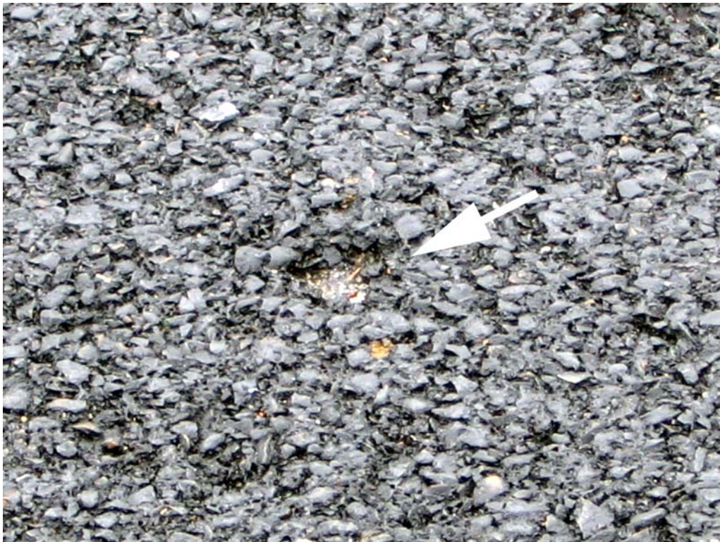
Figure 23. Hole at Station 56+80 (northbound direction).
