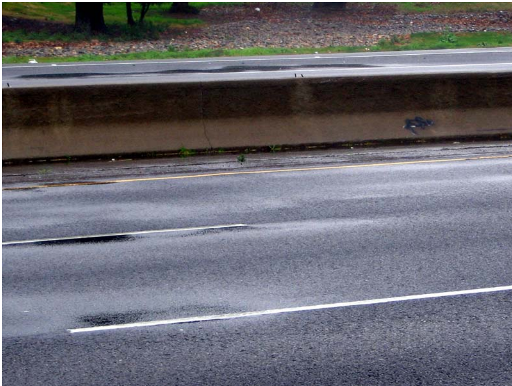
Figure 10. Ponding between Station 51+00 and Station 51+60 (inside lanes, southbound).
