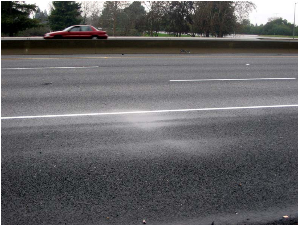
Figure 14. Reflection cracking between Station 51+00 and 52+00 (northbound lanes).
