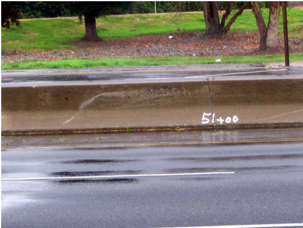
Figure 8. Ponding at Station 51+00 (inside lanes, southbound).
